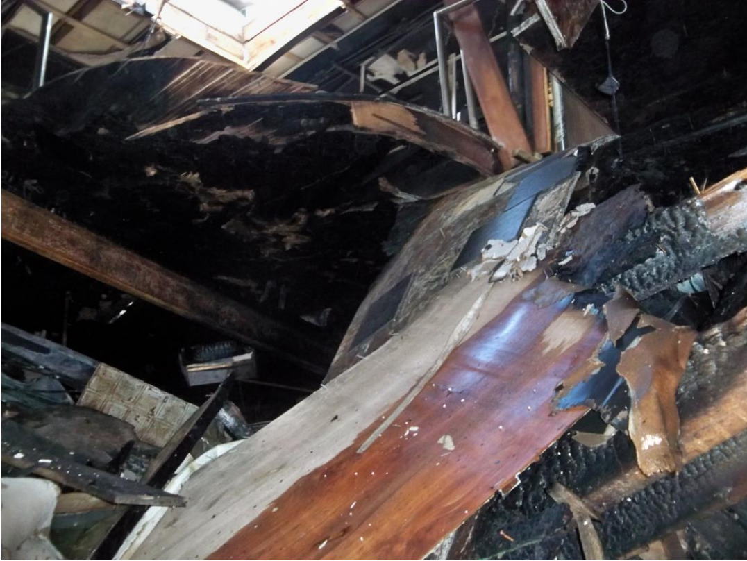
Photograph 7 - area of second-floor collapse within the building.
