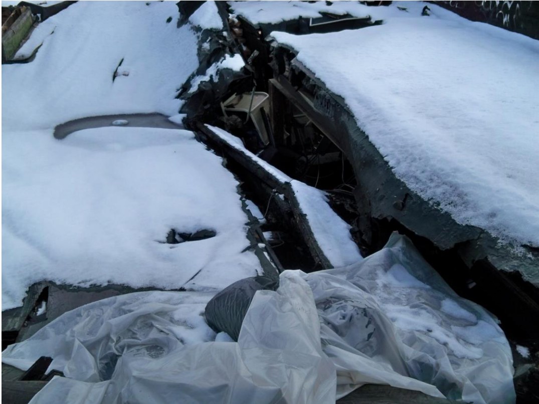
Photograph 5 - area of partial roof collapse and lateral displacement between main building and rear additions.
