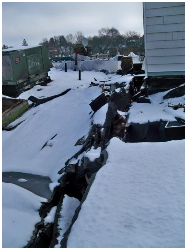
Photograph 4 - area of partial roof collapse and lateral displacement between main building and rear additions.
