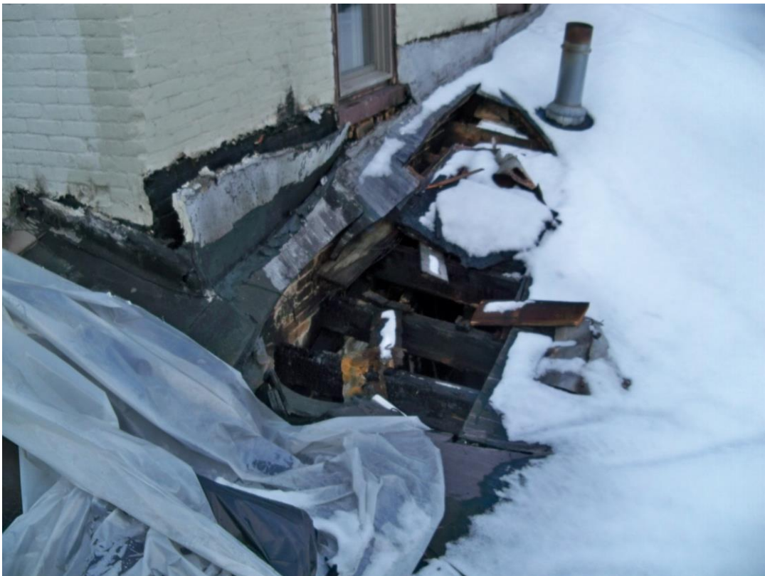
Photograph 6 - area of fire damaged roof and partial collapse at southwest corner of building.
