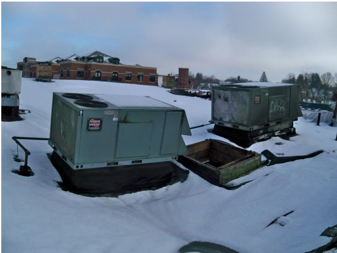
Photograph 2 - portion of partially collapsed roof where existing HVAC units are present.
