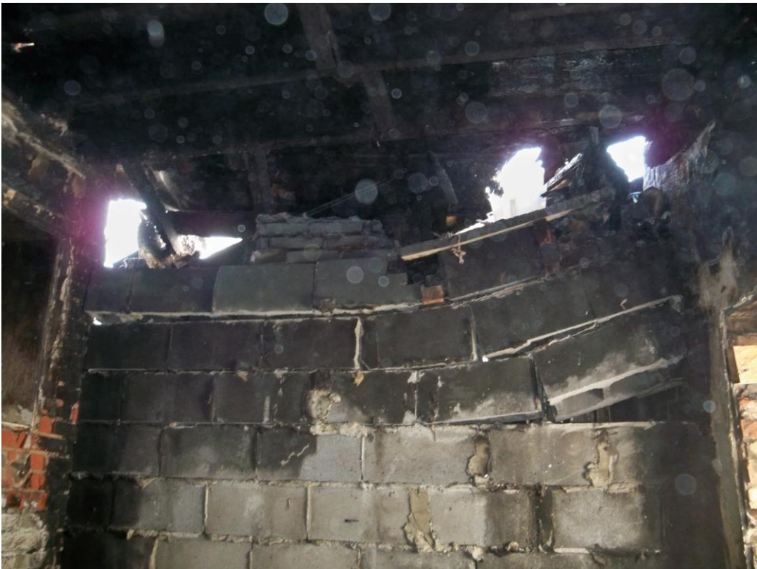
Photograph 8 - partial wall collapse at southwest corner of building.
